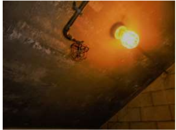
0001084e 4/24/2018 Sprinkler head and interior lighting First floor, elevator machine room
