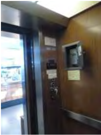
0001041a 4/24/2018 Elevator control panel and emergency phone Elevator
