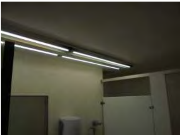
0001081e 4/24/2018 Interior lighting Second floor, men's restroom
