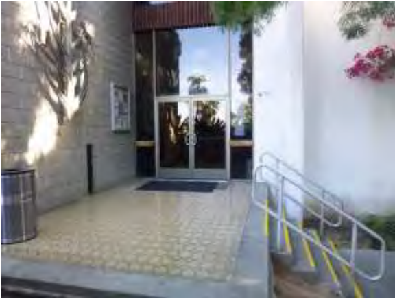
0001025a 4/24/2018 Entrance doors with door operator and damaged tile South entrance
