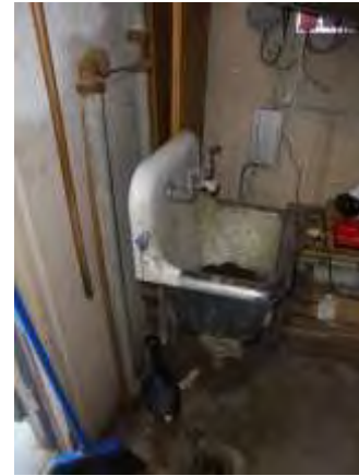
0002002e 4/24/2018 Service sink Mechanical/tool storage room
