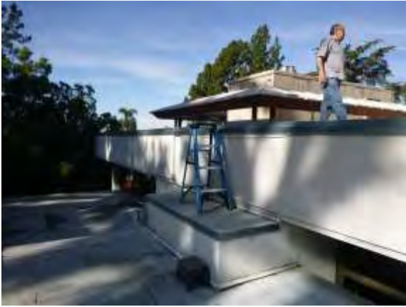
0001038a 4/24/2018 Missing fixed ladder Roof, east side
