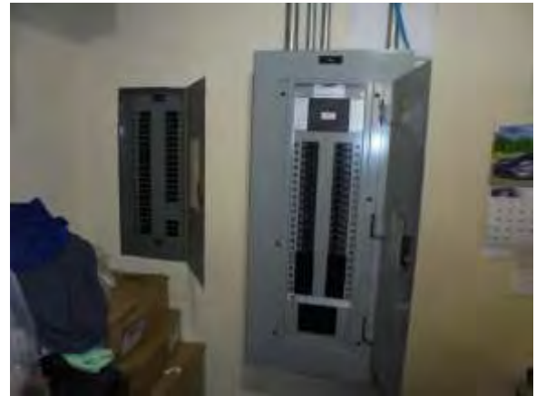
0001098e 4/24/2018 Panelboards First floor, custodial closet
