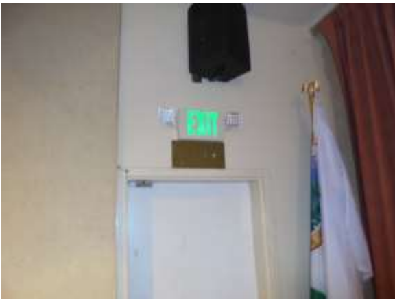
0001075e 4/24/2018 Exit sign and emergency light Second floor, conference room
