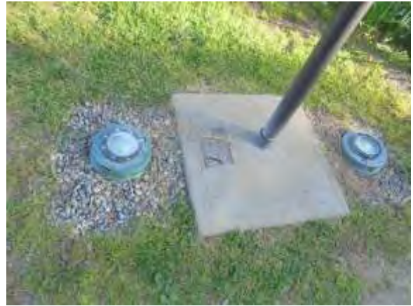
0001013e 4/24/2018 Exterior lighting Site
