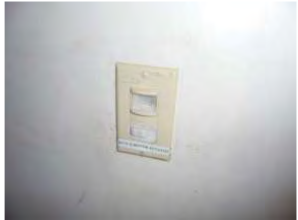
0002023e 4/24/2018 Occupancy sensor Women's restroom
