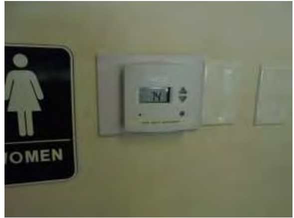
0002021e 4/24/2018 Digital thermostat Main room
