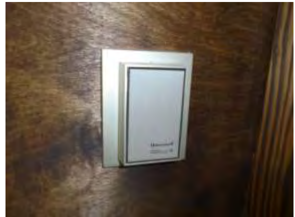
0001052e 4/24/2018 Honeywell thermostat Second floor, study room
