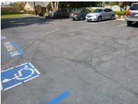
0002006a 4/24/2018 Cracked asphalt pavement Parking lot, west side of building
