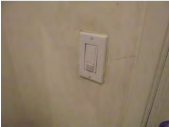
0002020e 4/24/2018 Occupancy sensor Men's restroom
