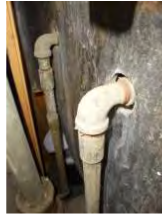
0002008e 4/24/2018 Original supply piping Mechanical/tool storage room
