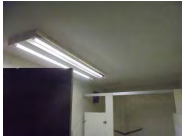
0001044e 4/24/2018 Interior lighting Second floor, men's restroom
