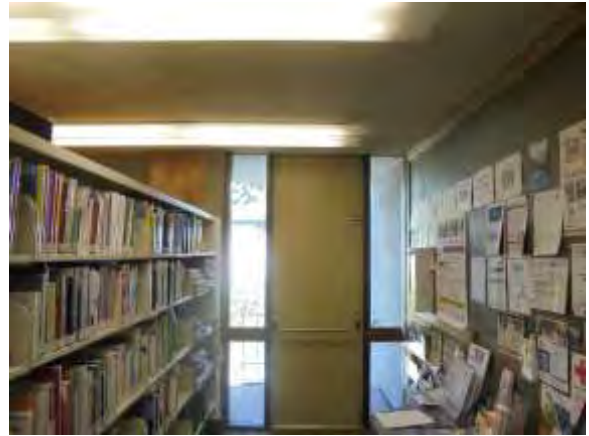
0001058e 4/24/2018 Lack of exit sign and emergency light Second floor, reading room
