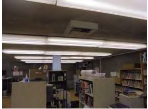
0001104e 4/24/2018 Interior lighting First floor, workroom
