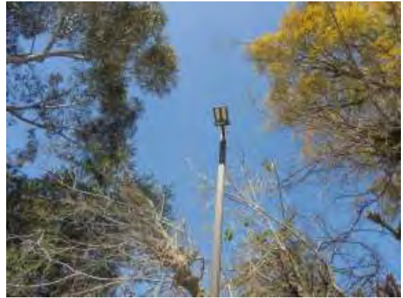
0002016e 4/24/2018 Exterior lighting Site
