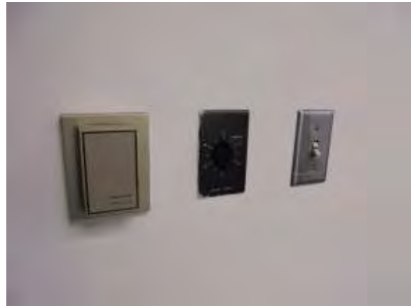
0001068e 4/24/2018 Honeywell thermostat and light switch Second floor, director's office
