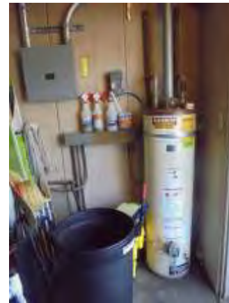
0002004e 4/24/2018 Water heater Mechanical/tool storage room
