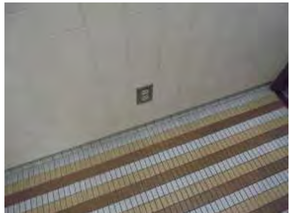
0001082e 4/24/2018 Non-GFCI receptacle Second floor, men's restroom
