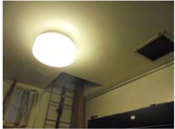
0001040e 4/24/2018 Interior lighting Second floor, IT room
