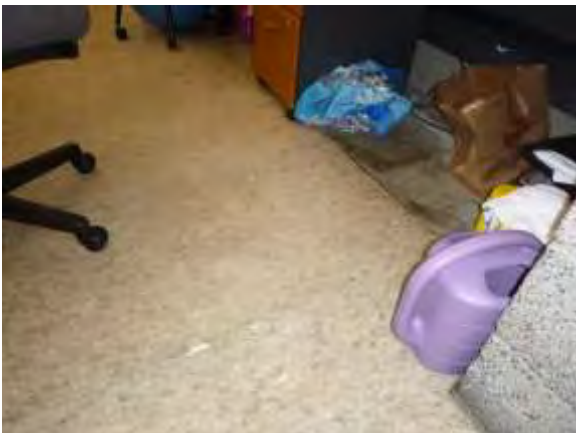
0001045a 4/24/2018 Worn vinyl tile floor Second floor, breakroom/circulation room
