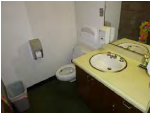
0001044a 4/24/2018 Countertop sink and low flow toilet with tank Second floor, director's office bathroom
