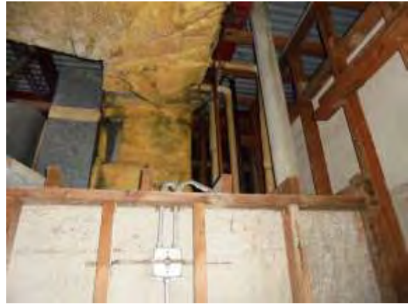
0001050e 4/24/2018 Possible asbestos pipe insulation and duct insulation Second floor, attic area
