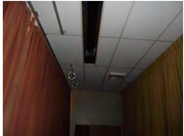
0001074e 4/24/2018 Interior lighting Second floor, conference room
