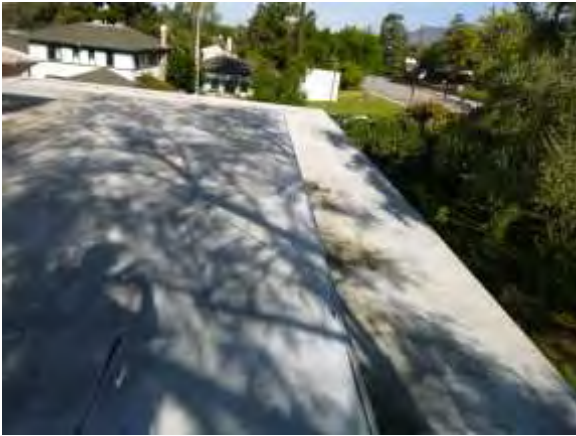
0001034a 4/24/2018 Roll asphalt roof with exposed seam Roof, north side looking west
