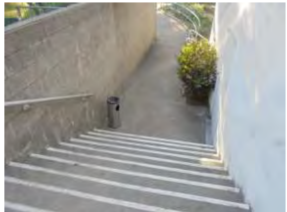
0001009e 4/24/2018 Lack of exterior lighting Site
