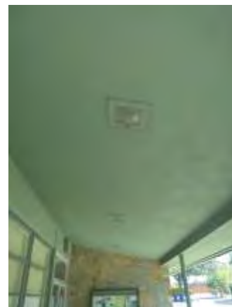
0002012e 4/24/2018 Exterior lighting Building exterior
