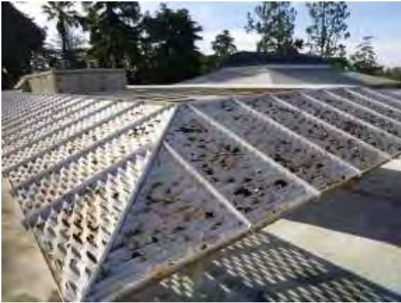
0001037a 4/24/2018 Corroded metal equipment screen Roof, north side, typical
