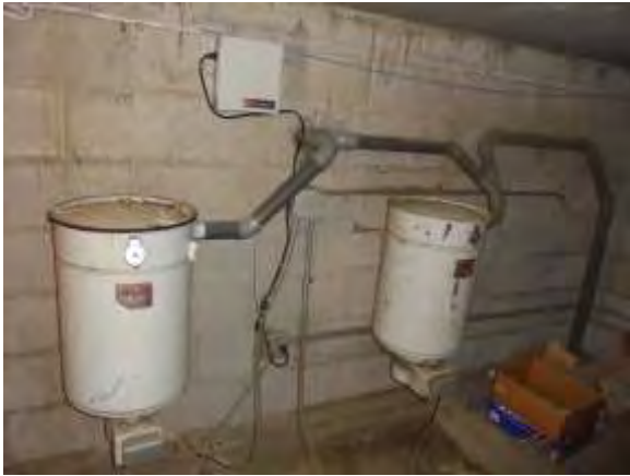
0001089e 4/24/2018 Inoperable vacuum system First floor, crawlspace
