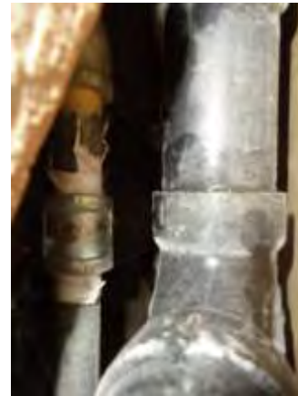
0002029e 4/24/2018 Plastic piping Main room, pipe chase
