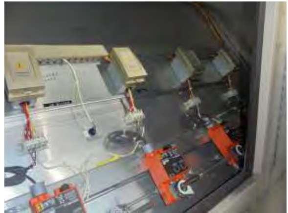
0001035e 4/24/2018 Electronic actuators for rooftop package unit #3 Roof
