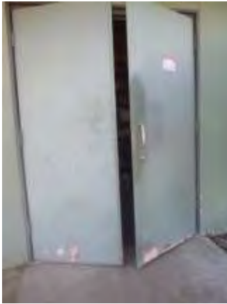
0002007a 4/24/2018 Mechanical room doors that are delaminated at the bottom Mechanical room, southwest side of building
