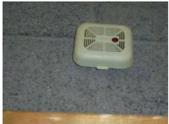
0001060e 4/24/2018 Local-only smoke detector Second floor, reading room
