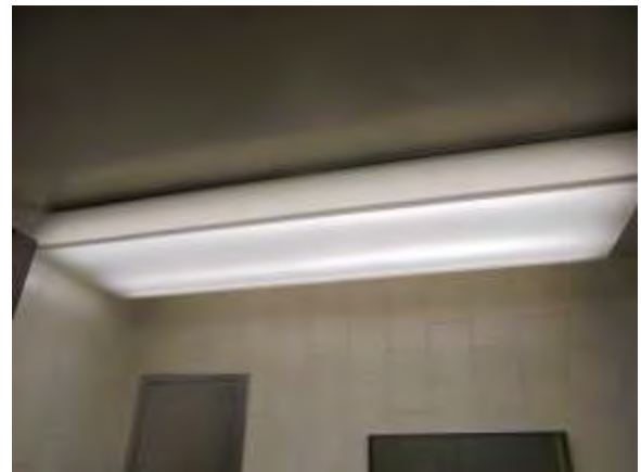
0001100e 4/24/2018 Interior lighting First floor, women's restroom
