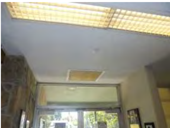
0002030e 4/24/2018 Interior lighting and lack of exit sign/emergency light Main room
