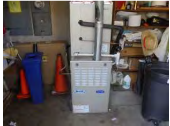
0002007e 4/24/2018 Furnace Mechanical/tool storage room
