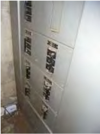
0001107e 4/24/2018 Switchboard First floor, exterior electrical room
