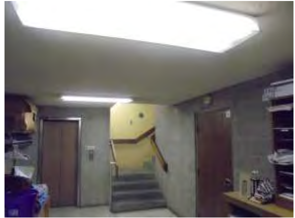
0001090e 4/24/2018 Local-only smoke detector and interior lighting First floor, corridor
