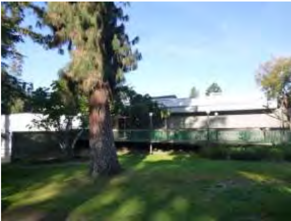
0001017a 4/24/2018 Northeast elevation and CMU and stucco siding Northeast side of building
