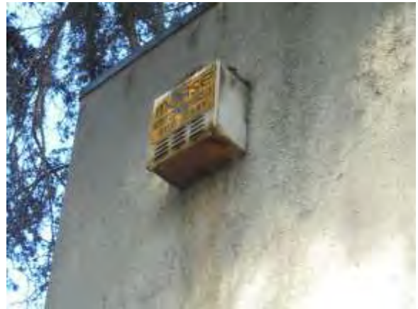
0001011e 4/24/2018 Aged alarm bell Building exterior
