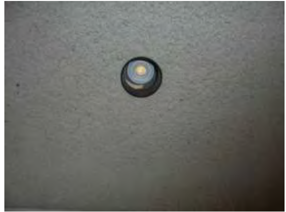
0001067e 4/24/2018 Interior lighting Second floor, director's office
