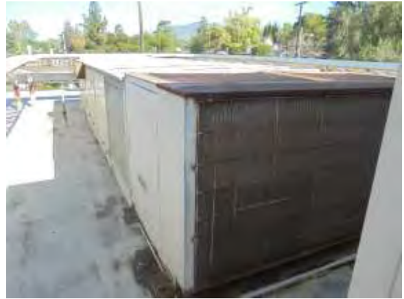
0001028e 4/24/2018 Inoperable rooftop package unit #1 Roof
