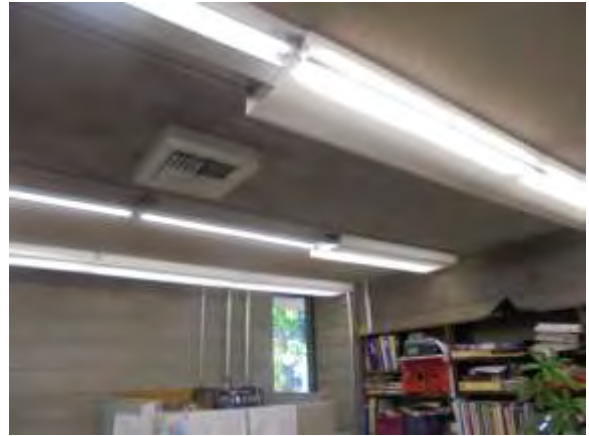
0001041e 4/24/2018 Interior lighting Second floor, circulation room
