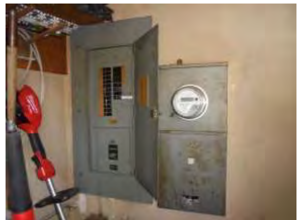
0002003e 4/24/2018 Panelboard and electrical meter Mechanical/tool storage room
