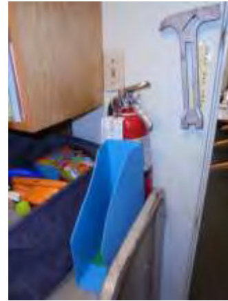
0002039e 4/24/2018 Fire extinguisher Staff room
