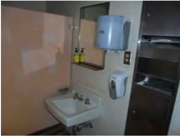
0001101e 4/24/2018 Non-GFCI receptacle First floor, men's restroom
