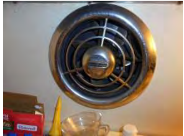
0001078e 4/24/2018 Exhaust fan Second floor, conference room
