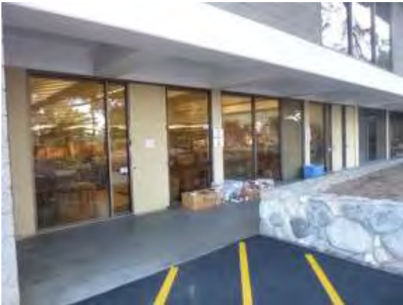
0001002a 4/24/2018 Single-pane windows, metal doors, structural concrete, and CMU First floor, south side
