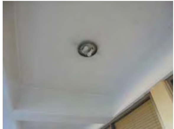
0001023e 4/24/2018 Exterior lighting Building exterior
