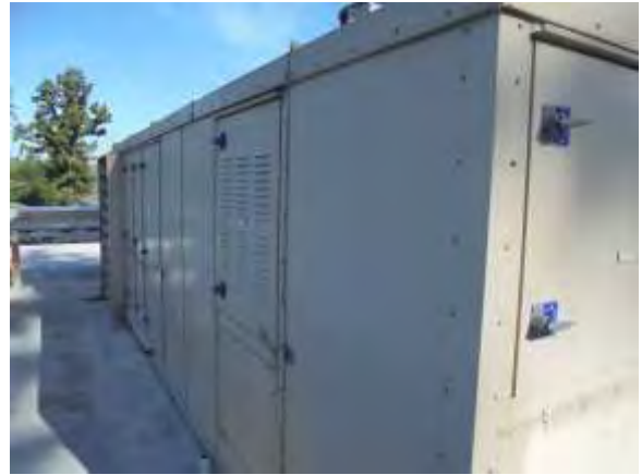
0001034e 4/24/2018 Rooftop package unit #3 Roof
