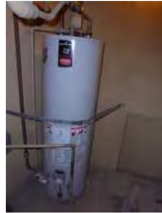
0001046e 4/24/2018 Water heater Second floor, custodial closet
