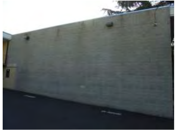
0001001e 4/24/2018 Exterior lighting Building exterior
