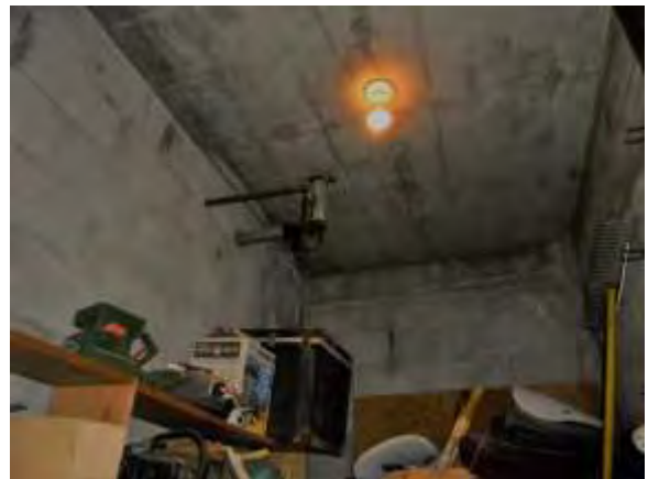
0001027e 4/24/2018 Sprinkler head and interior lighting First floor, tool storage room
