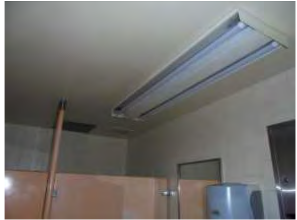
0001102e 4/24/2018 Interior lighting First floor, men's restroom
