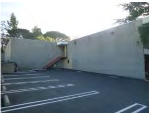
0001003a 4/24/2018 West elevation, fire escape with noncompliant handrails, and CMU Southwest elevation looking north
