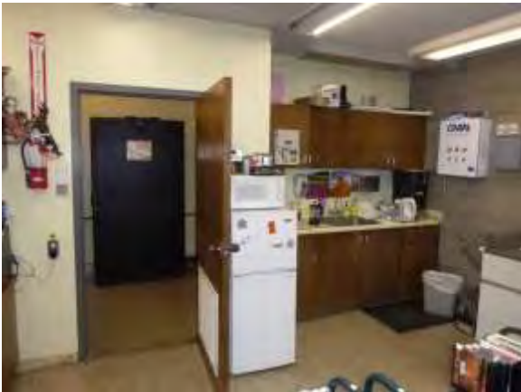
0001039a 4/24/2018 Old cabinets, knob door hardware, and 9- and 12-inch tile Second floor, east side rooms
