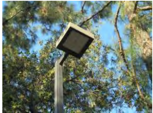
0001017e 4/24/2018 Exterior lighting Site
