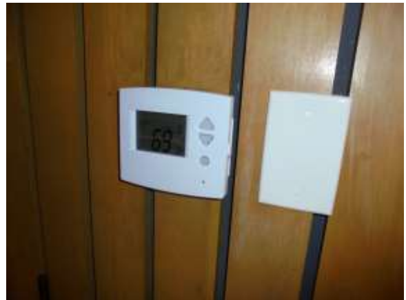
0001076e 4/24/2018 Digital thermostat Second floor, conference room
