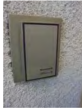
0001055e 4/24/2018 Honeywell thermostat Second floor, reading room
