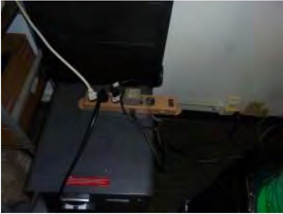
0002040e 4/24/2018 Electrical outlet strip Staff room
