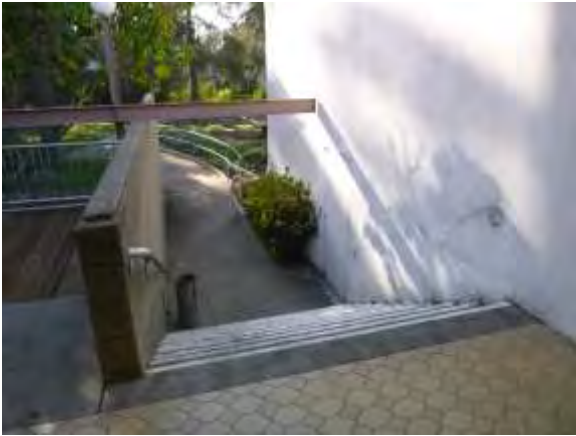
0001016a 4/24/2018 Noncompliant and missing handrails and stucco siding East side steps at main entrance
