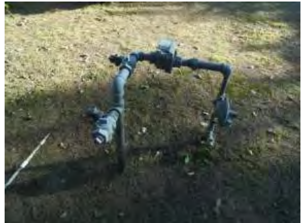
0001014e 4/24/2018 Gas regulator Site
