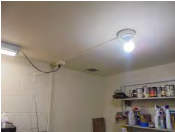
0001097e 4/24/2018 Interior lighting First floor, custodial closet
