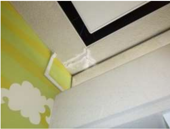
0001050a 4/24/2018 Ceiling damage Second floor, southeast side
