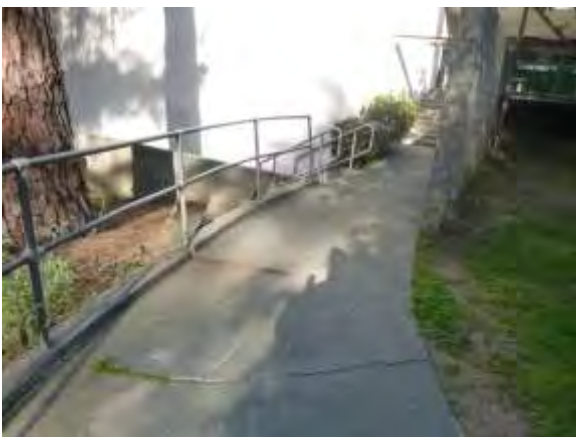
0001021a 4/24/2018 Cracked, sunken sidewalk and leaning and corroded handrails East side of building
