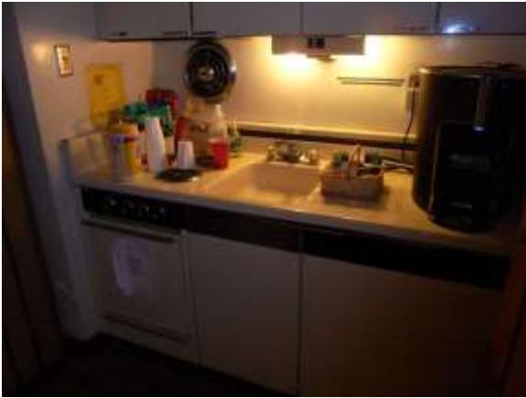
0001077e 4/24/2018 Lack of fire suppression Second floor, conference room
