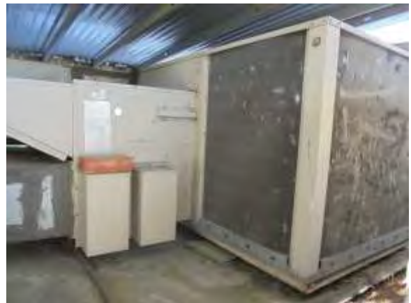
0001036e 4/24/2018 Rooftop package unit #4 Roof
