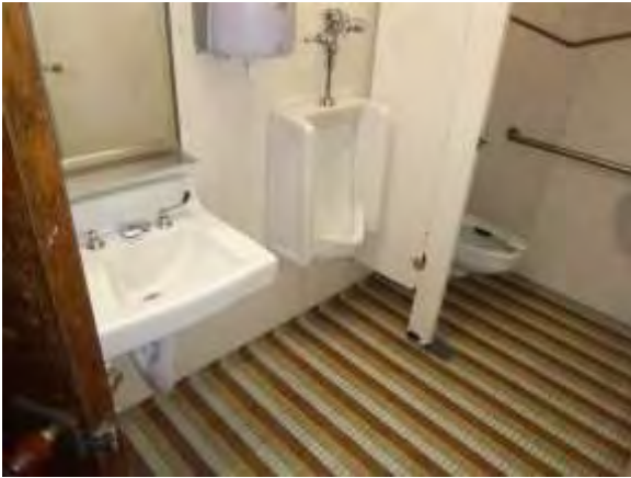
0001049a 4/24/2018 Restroom fixtures and finishes, door that opens in, and knob hardware Second floor, men's restroom
