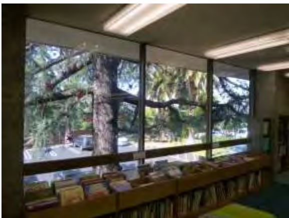
0001054a 4/24/2018 Single-pane fixed windows, some of which rattle Second floor, library, south side
