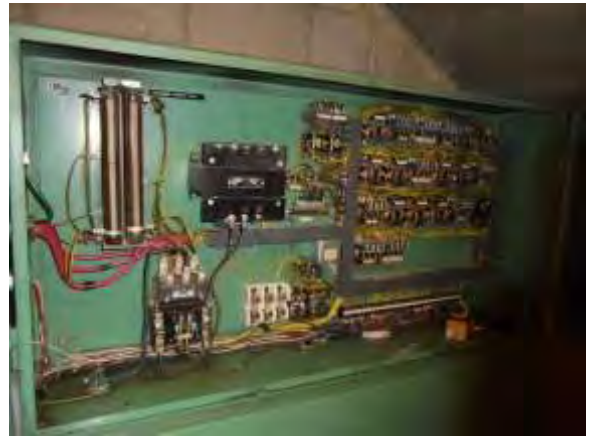
0001086e 4/24/2018 Elevator controller First floor, elevator machine room
