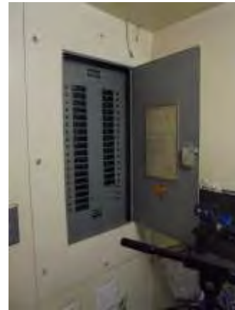
0001080e 4/24/2018 Panelboard Second floor, conference room closet
