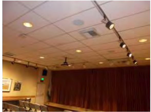
0001073e 4/24/2018 Interior lighting Second floor, conference room
