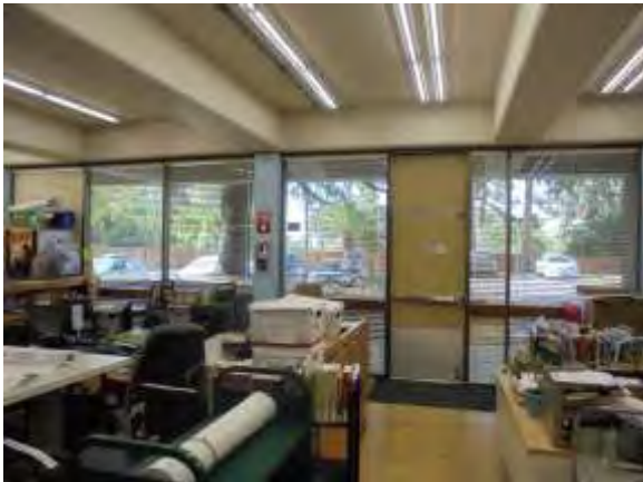
0001105e 4/24/2018 Lack of exit signage and emergency light First floor, workroom
