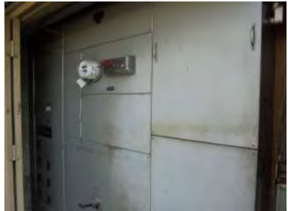
0001106e 4/24/2018 Switchboard First floor, exterior electrical room
