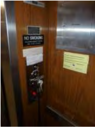
0001083e 4/24/2018 Car operating panel Elevator cab
