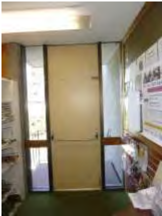
0001053a 4/24/2018 Fire escape exit door, panic hardware, and missing LED exit sign Second floor, library, west side
