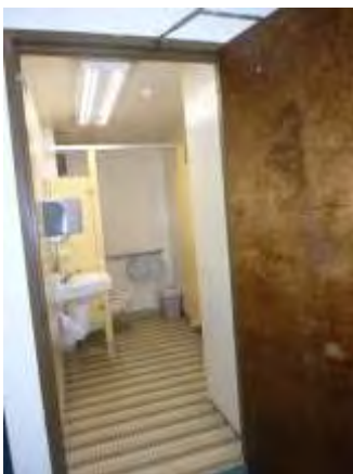
0001048a 4/24/2018 Scarred wood door and ceramic tile floor and walls Second floor, women's restroom
