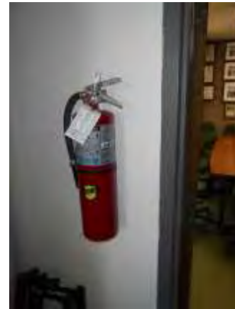
0001065e 4/24/2018 Fire extinguisher Second floor, director's office, secretary
