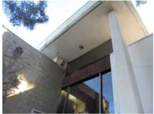
0001022e 4/24/2018 Exterior lighting Building exterior
