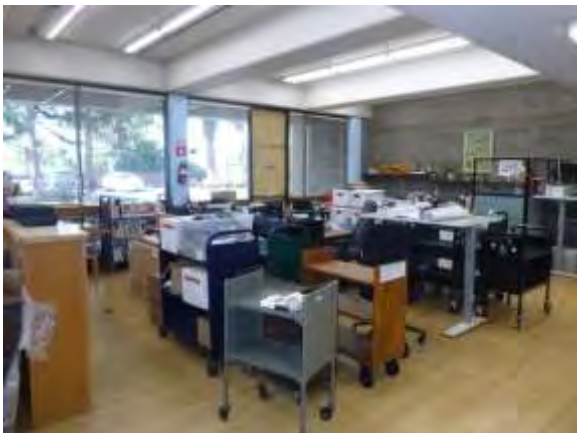
0001069a 4/24/2018 Laminate floor, painted ceiling, and missing LED exit sign First floor, technical services room
