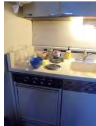
0001094e 4/24/2018 Lack of fire suppression First floor, staff lounge
