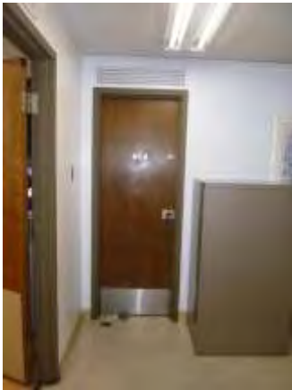
0001071a 4/24/2018 Narrow restroom entrance door, knob hardware, and lack of Braille First floor, hallway
