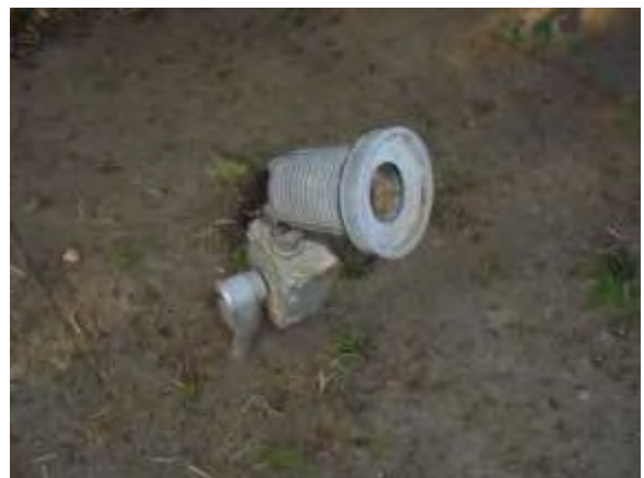
0001021e 4/24/2018 Exterior lighting Site
