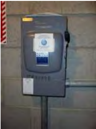
0001085e 4/24/2018 Electrical disconnect switch First floor, elevator machine room
