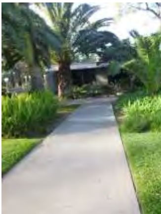
0001009a 4/24/2018 Concrete sidewalk repair, lack of handrails, and landscaping North side access from curb cut
