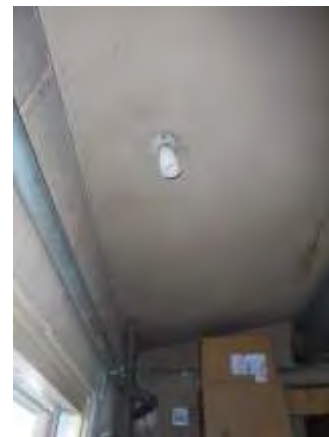
0002006e 4/24/2018 Interior lighting Mechanical/tool storage room
