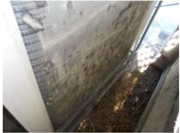
0001037e 4/24/2018 Coils for rooftop package unit #4 Roof
