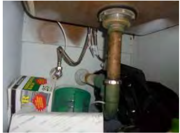
0002027e 4/24/2018 Supply and drain piping Staff room
