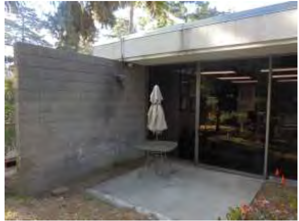
0001004e 4/24/2018 Exterior lighting Building exterior
