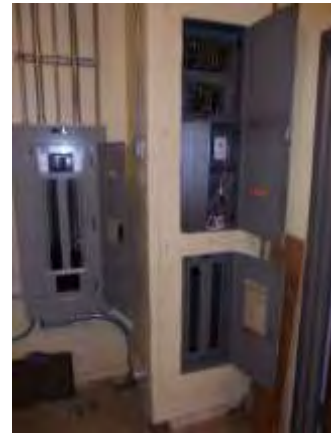
0001039e 4/24/2018 Panelboards Second floor, IT room
