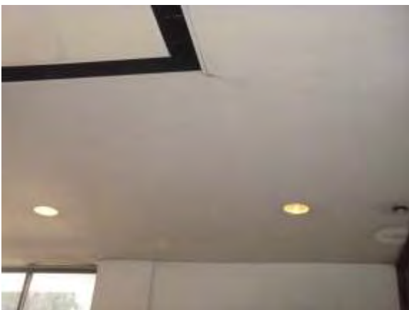
0001051a 4/24/2018 Cracks in painted ceiling and some staining Second floor, library, east side
