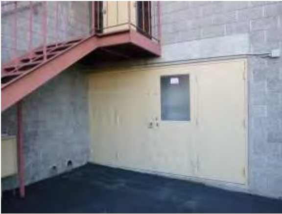
0001004a 4/24/2018 Old metal doors to electrical and mechanical area and CMU exterior First floor, west side
