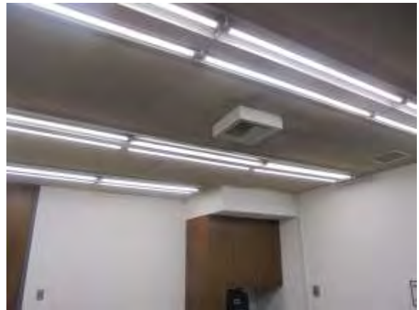
0001072e 4/24/2018 Interior lighting Second floor, passport office
