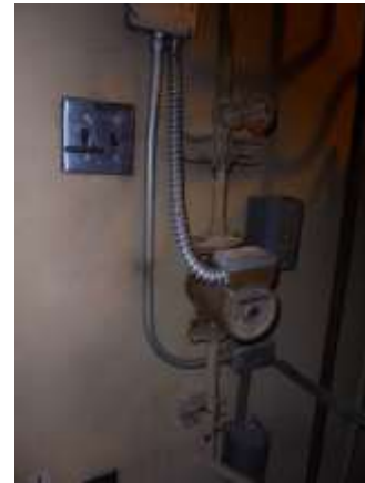
0001047e 4/24/2018 Circulation pump Second floor, custodial closet
