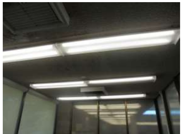
0001051e 4/24/2018 Interior lighting Second floor, study room
