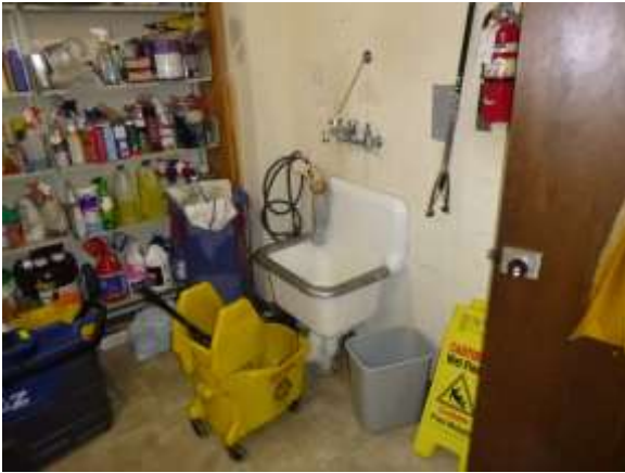
0001067a 4/24/2018 Service sink, roll vinyl floor, and knob door hardware First floor, custodial closet
