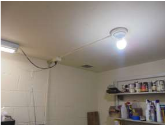
0001097e 4/24/2018 Interior lighting First floor, custodial closet
