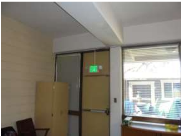
0001093e 4/24/2018 Exit sign and emergency light First floor, staff lounge
