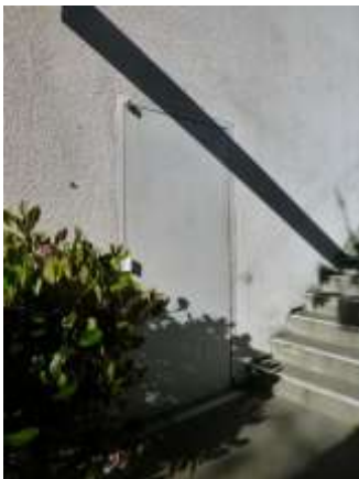
0001027a 4/24/2018 Conference room exit door and ADA entrance with some corrosion Split-level conference room, east side
