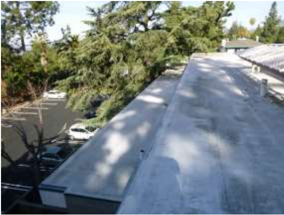
0001031a 4/24/2018 Roll asphalt roofs and metal screen Roof, south side looking west
