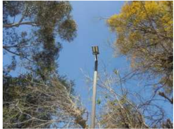
0002016e 4/24/2018 Exterior lighting Site
