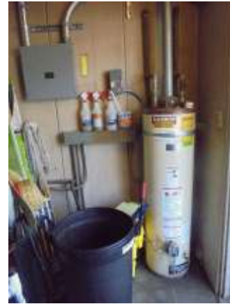
0002004e 4/24/2018 Water heater Mechanical/tool storage room
