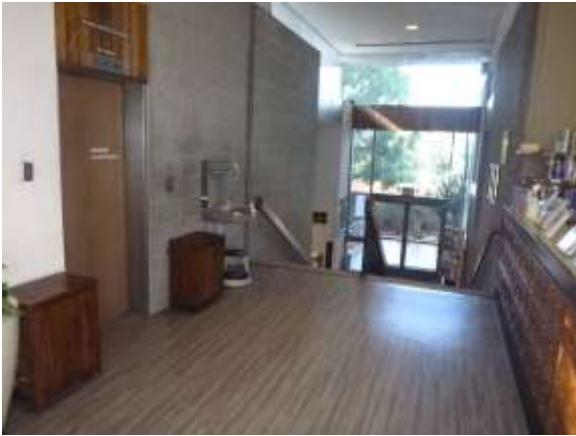
0001040a 4/24/2018 Elevator, drinking fountain, laminate floor, and step handrails Second floor, southeast side
