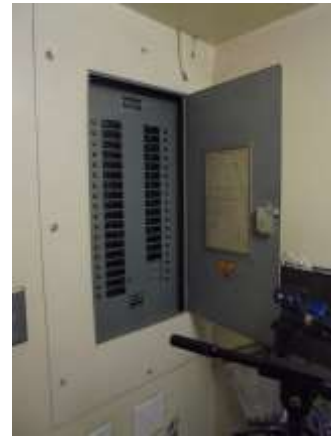
0001080e 4/24/2018 Panelboard Second floor, conference room closet
