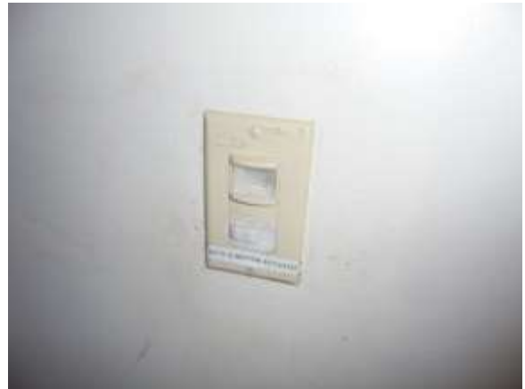
0002023e 4/24/2018 Occupancy sensor Women's restroom
