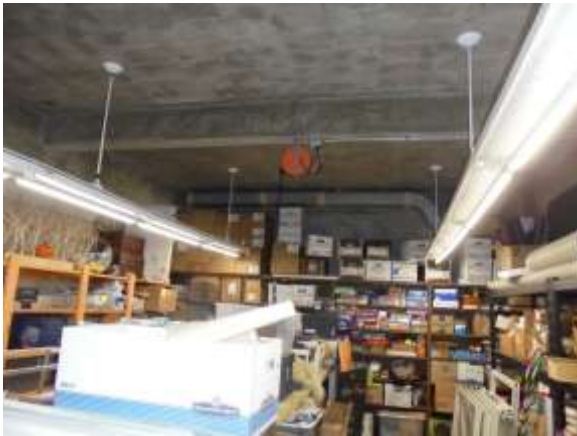
0001091e 4/24/2018 Interior lighting First floor, book storage room
