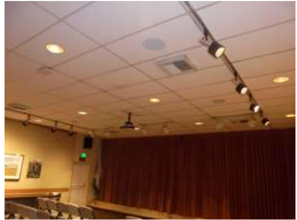
0001073e 4/24/2018 Interior lighting Second floor, conference room
