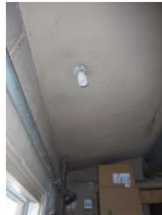
0002006e 4/24/2018 Interior lighting Mechanical/tool storage room
