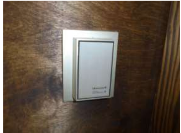
0001052e 4/24/2018 Honeywell thermostat Second floor, study room
