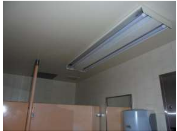
0001102e 4/24/2018 Interior lighting First floor, men's restroom
