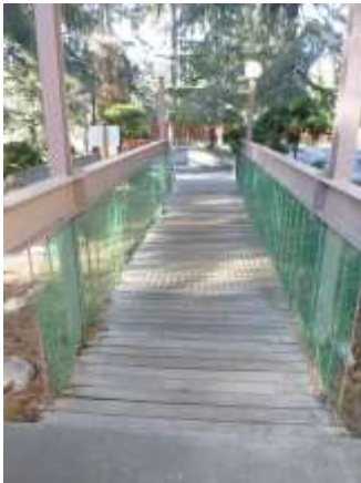
0001020a 4/24/2018 Damaged, rotted, uneven wood planks on pedestrian bridge Southeast side of facility
