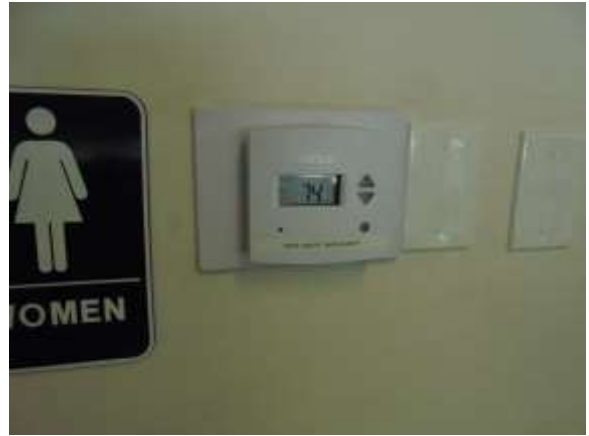
0002021e 4/24/2018 Digital thermostat Main room
