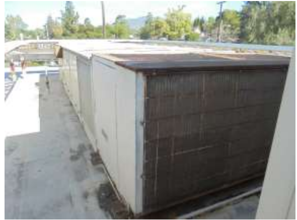
0001028e 4/24/2018 Inoperable rooftop package unit #1 Roof
