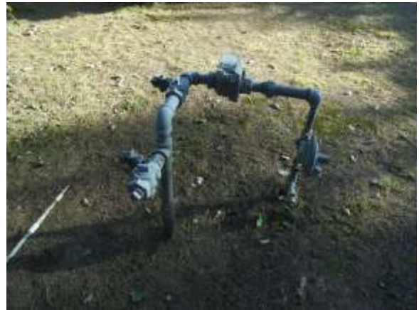
0001014e 4/24/2018 Gas regulator Site
