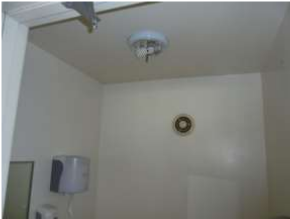
0002022e 4/24/2018 Exhaust fan and interior lighting Women's restroom
