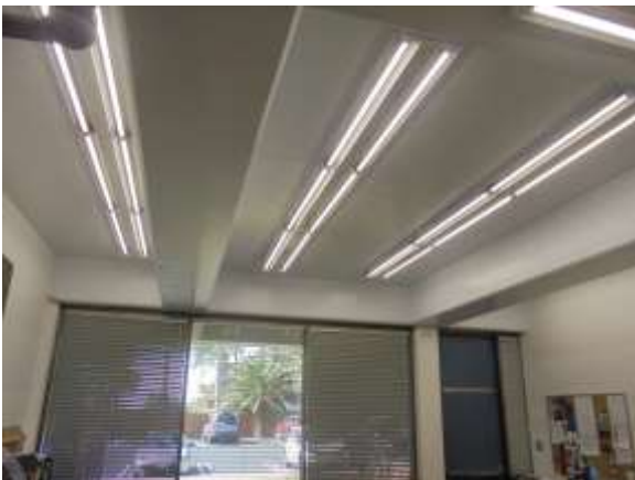
0001099e 4/24/2018 Interior lighting First floor, office
