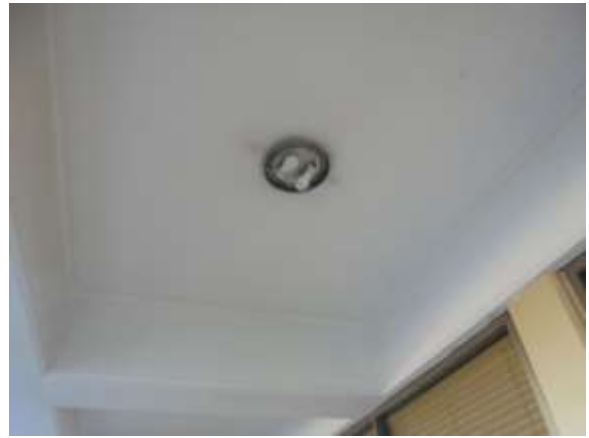
0001023e 4/24/2018 Exterior lighting Building exterior
