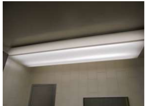
0001100e 4/24/2018 Interior lighting First floor, women's restroom
