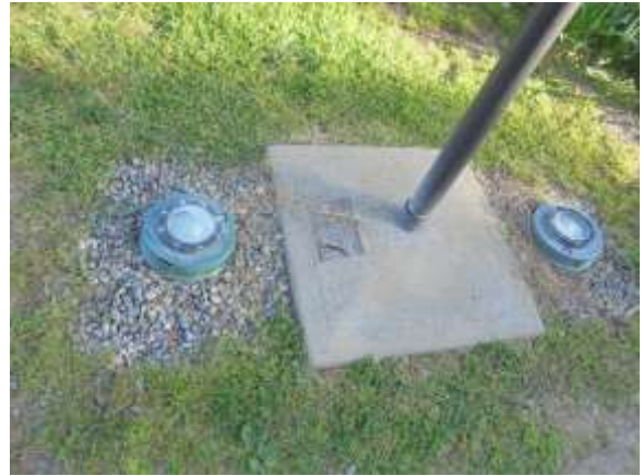
0001013e 4/24/2018 Exterior lighting Site
