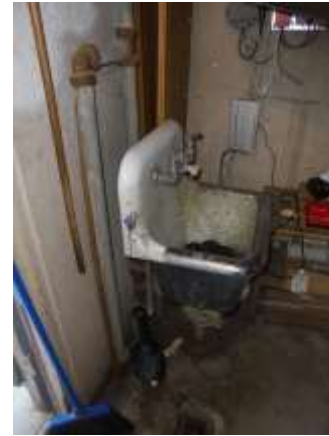
0002002e 4/24/2018 Service sink Mechanical/tool storage room
