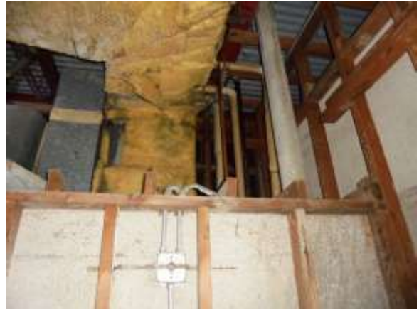
0001050e 4/24/2018 Possible asbestos pipe insulation and duct insulation Second floor, attic area
