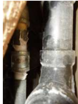
0002029e 4/24/2018 Plastic piping Main room, pipe chase
