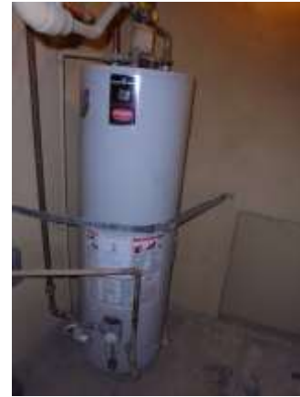
0001046e 4/24/2018 Water heater Second floor, custodial closet
