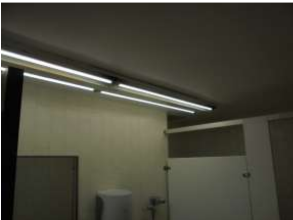
0001081e 4/24/2018 Interior lighting Second floor, men's restroom
