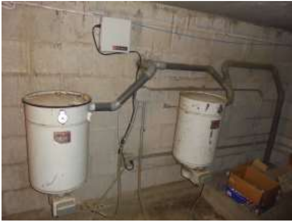
0001089e 4/24/2018 Inoperable vacuum system First floor, crawlspace
