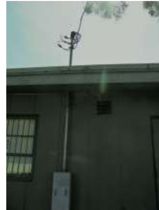
0002001e 4/24/2018 Electrical service drop Building exterior
