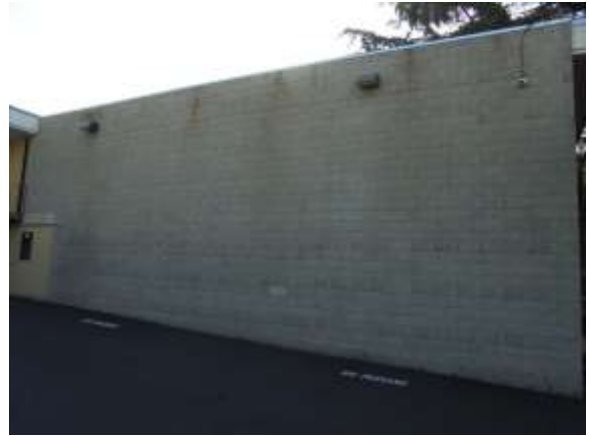
0001001e 4/24/2018 Exterior lighting Building exterior
