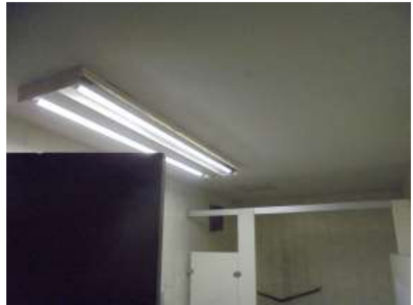
0001044e 4/24/2018 Interior lighting Second floor, men's restroom
