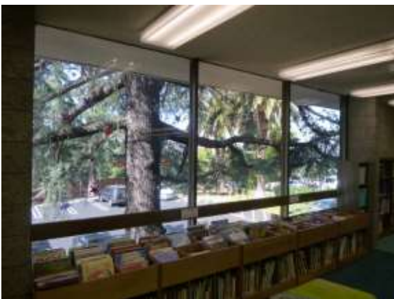
0001054a 4/24/2018 Single-pane fixed windows, some of which rattle Second floor, library, south side
