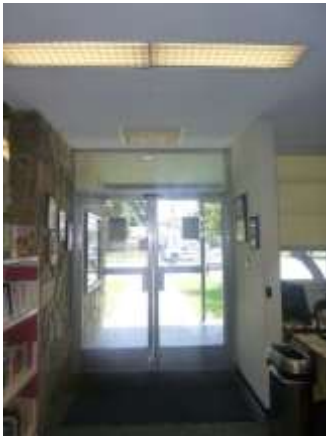
0002017a 4/24/2018 Missing LED exit signage East side entrance/exit
