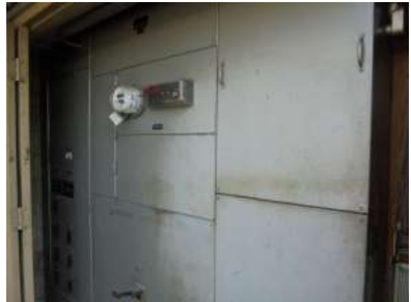
0001106e 4/24/2018 Switchboard First floor, exterior electrical room
