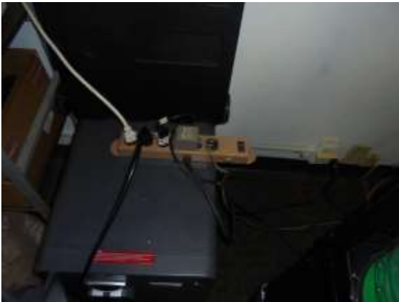
0002040e 4/24/2018 Electrical outlet strip Staff room
