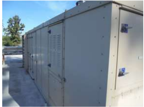
0001034e 4/24/2018 Rooftop package unit #3 Roof
