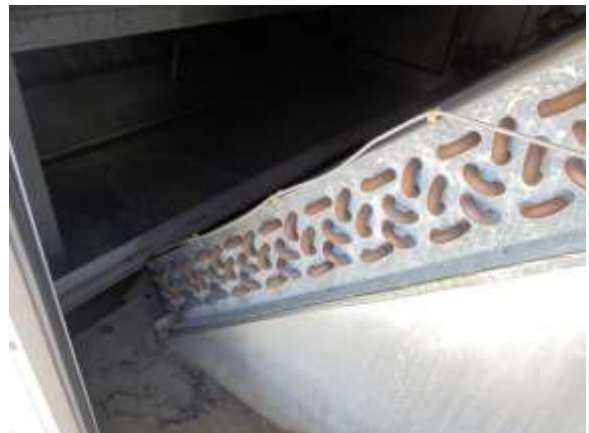
0001033e 4/24/2018 Coil section of rooftop package unit #2 Roof
