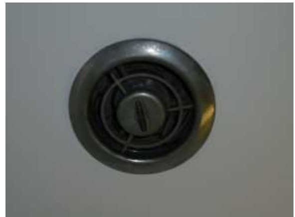
0001069e 4/24/2018 Exhaust fan Second floor, director's office, restroom
