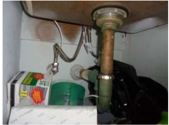
0002027e 4/24/2018 Supply and drain piping Staff room
