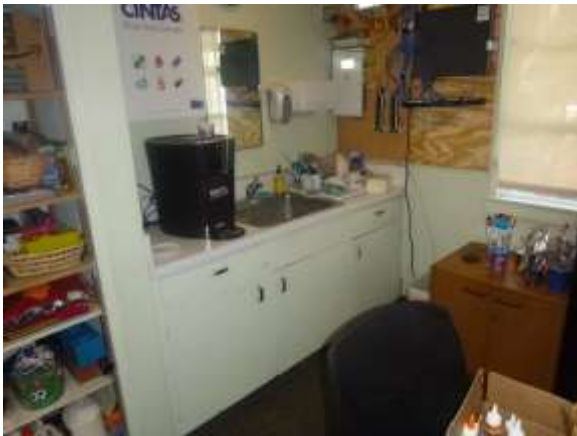
0002012a 4/24/2018 Old cabinets, sink, and carpet Staff room
