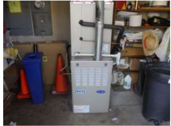
0002007e 4/24/2018 Furnace Mechanical/tool storage room
