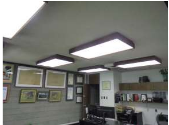
0001066e 4/24/2018 Interior lighting Second floor, director's office
