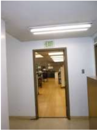
0001070a 4/24/2018 Nonilluminating exit sign and missing Braille signage First floor, hallway
