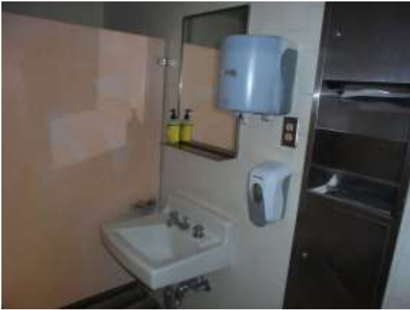
0001101e 4/24/2018 Non-GFCI receptacle First floor, men's restroom
