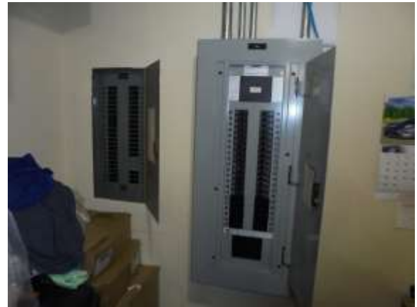
0001098e 4/24/2018 Panelboards First floor, custodial closet
