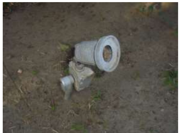
0001021e 4/24/2018 Exterior lighting Site
