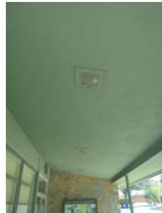
0002012e 4/24/2018 Exterior lighting Building exterior
