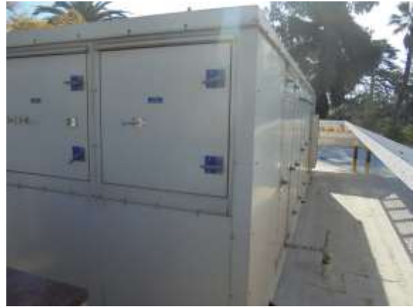
0001031e 4/24/2018 Rooftop package unit #2 Roof
