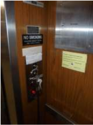
0001083e 4/24/2018 Car operating panel Elevator cab
