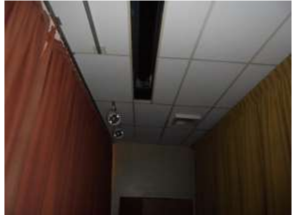
0001074e 4/24/2018 Interior lighting Second floor, conference room
