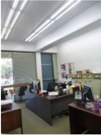
0001068a 4/24/2018 Carpet, missing LED exit sign, and painted ceiling First floor, office
