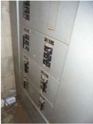
0001107e 4/24/2018 Switchboard First floor, exterior electrical room
