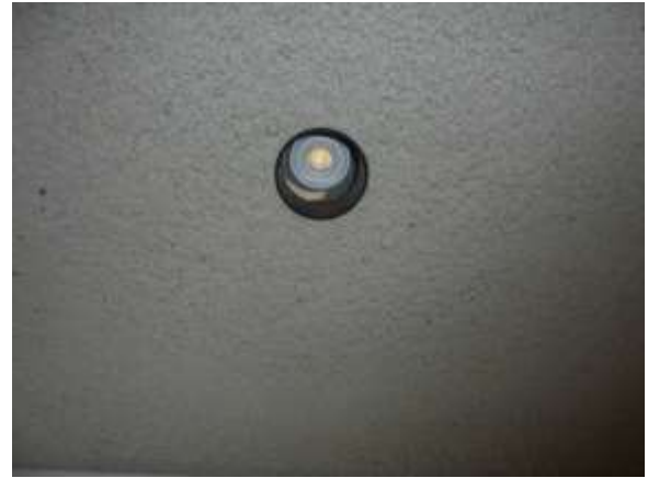
0001067e 4/24/2018 Interior lighting Second floor, director's office
