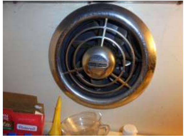
0001078e 4/24/2018 Exhaust fan Second floor, conference room
