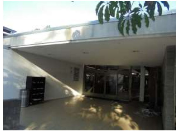
0001008e 4/24/2018 Exterior lighting Building exterior
