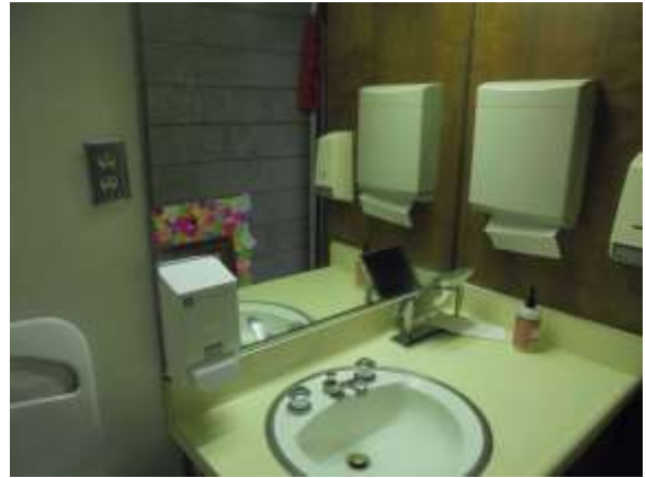
0001070e 4/24/2018 Non-GFCI receptacle Second floor, director's office, restroom
