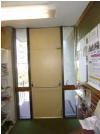
0001053a 4/24/2018 Fire escape exit door, panic hardware, and missing LED exit sign Second floor, library, west side
