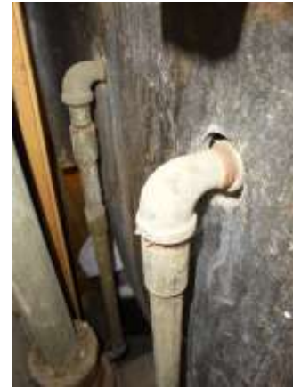
0002008e 4/24/2018 Original supply piping Mechanical/tool storage room
