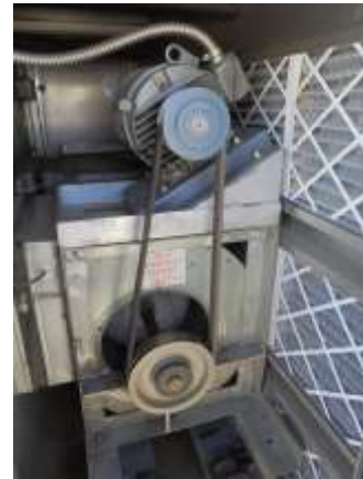
0001032e 4/24/2018 Fan section of rooftop package unit #2 Roof
