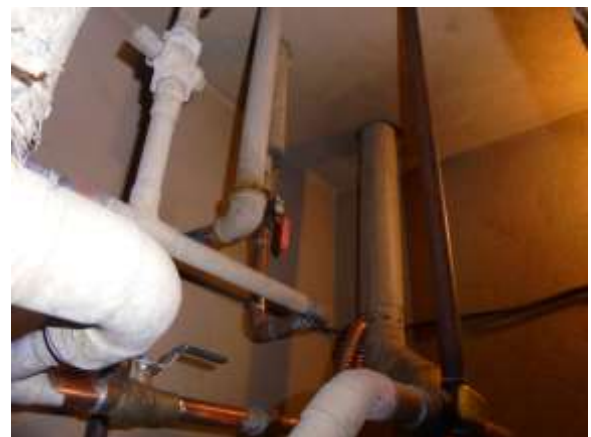
0001048e 4/24/2018 Piping Second floor, custodial closet
