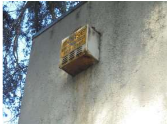
0001011e 4/24/2018 Aged alarm bell Building exterior
