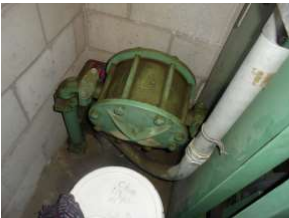
0001087e 4/24/2018 Silencer First floor, elevator machine room
