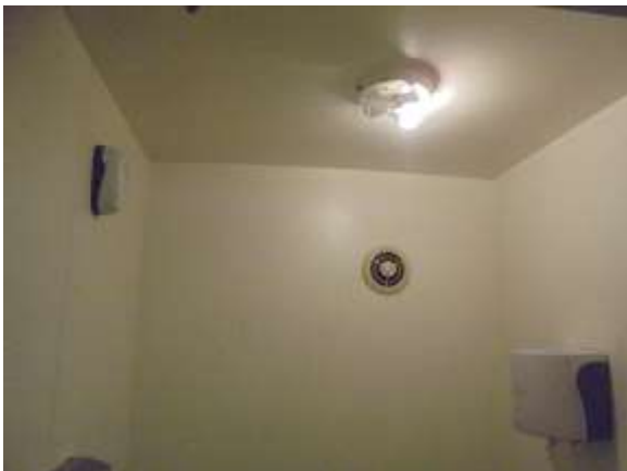
0002018e 4/24/2018 Exhaust fan and interior lighting Men's restroom
