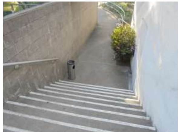
0001009e 4/24/2018 Lack of exterior lighting Site
