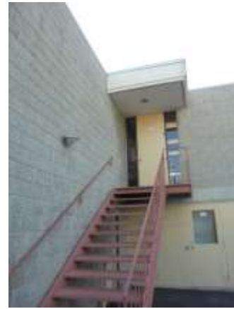
0001002e 4/24/2018 Exterior lighting Building exterior
