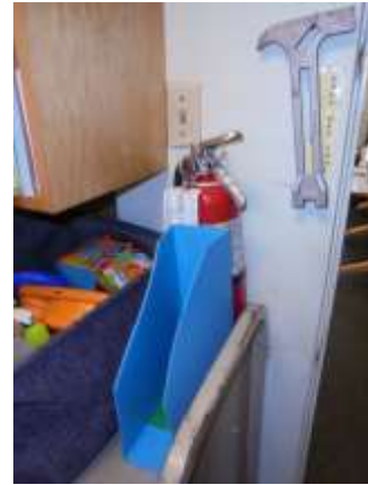
0002039e 4/24/2018 Fire extinguisher Staff room
