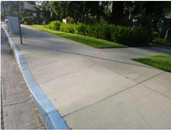
0001008a 4/24/2018 Curb cut in municipal sidewalk with steep slope Mariposa Street, north side of facility
