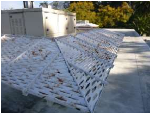
0001032a 4/24/2018 Metal equipment screens with some corrosion Roof, south side equipment screen
