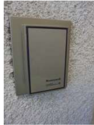
0001055e 4/24/2018 Honeywell thermostat Second floor, reading room
