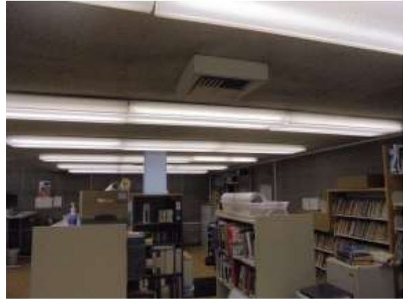
0001104e 4/24/2018 Interior lighting First floor, workroom
