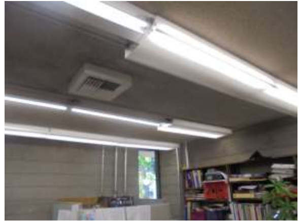
0001041e 4/24/2018 Interior lighting Second floor, circulation room
