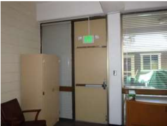
0001066a 4/24/2018 LED exit signage and panic door hardware First floor, breakroom
