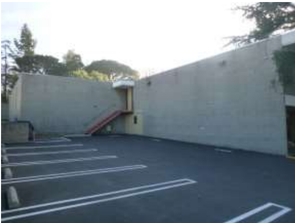
0001003a 4/24/2018 West elevation, fire escape with noncompliant handrails, and CMU Southwest elevation looking north
