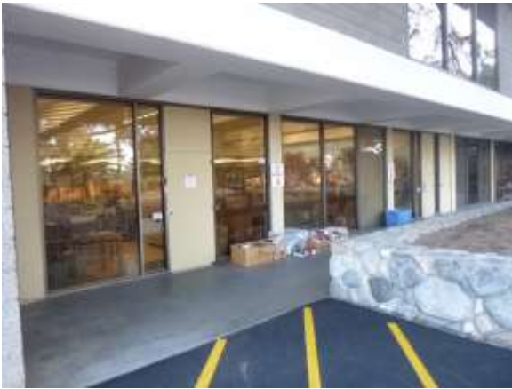
0001002a 4/24/2018 Single-pane windows, metal doors, structural concrete, and CMU First floor, south side
