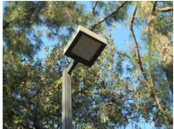
0001017e 4/24/2018 Exterior lighting Site
