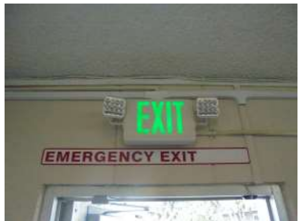
0002031e 4/24/2018 Exit sign and emergency light Main room
