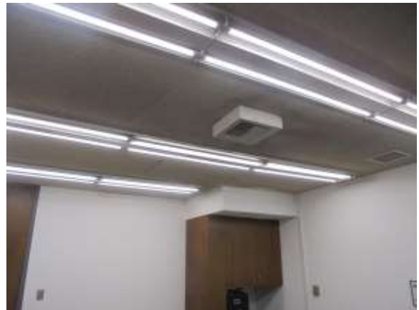
0001072e 4/24/2018 Interior lighting Second floor, passport office
