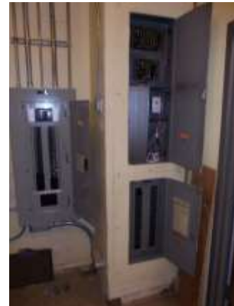
0001039e 4/24/2018 Panelboards Second floor, IT room
