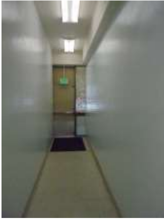
0001103e 4/24/2018 Exit sign and emergency light First floor, corridor
