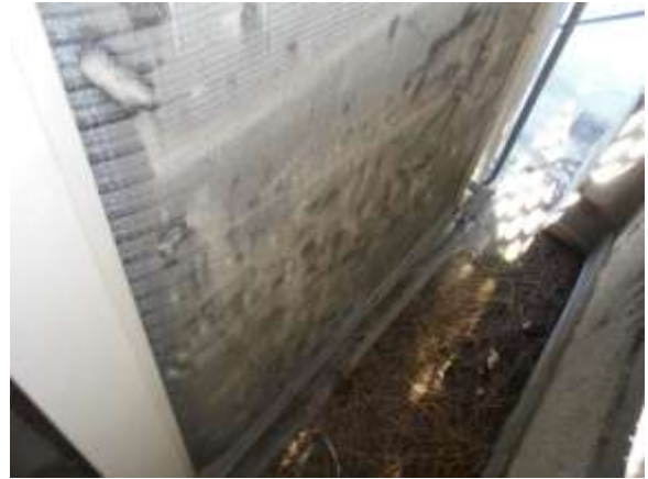
0001037e 4/24/2018 Coils for rooftop package unit #4 Roof
