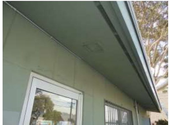
0002017e 4/24/2018 Exterior lighting Building exterior
