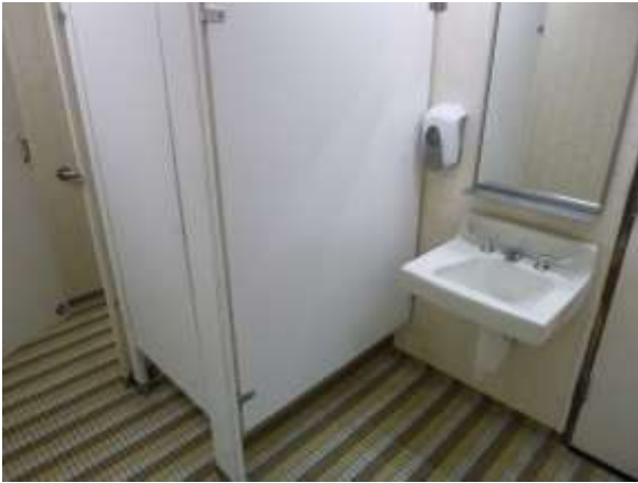
0001058a 4/24/2018 Ceramic tile floor and walls and old sink and partition Split-level women's restroom
