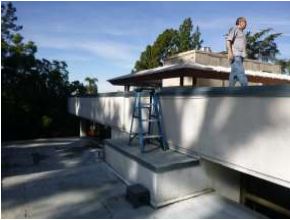
0001038a 4/24/2018 Missing fixed ladder Roof, east side
