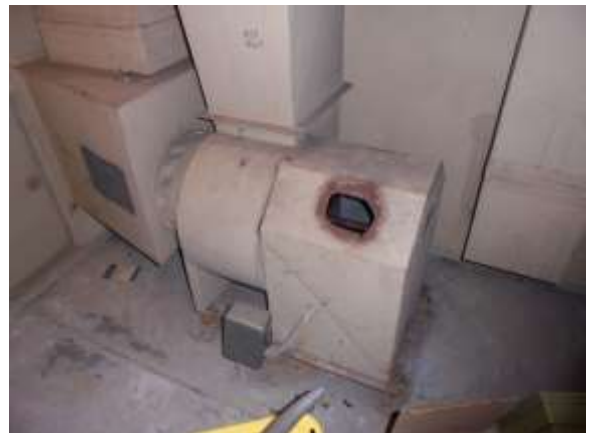
0001045e 4/24/2018 Restroom exhaust fan Second floor, custodial closet
