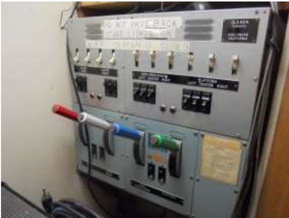
0001079e 4/24/2018 Lighting controls Second floor, conference room closet
