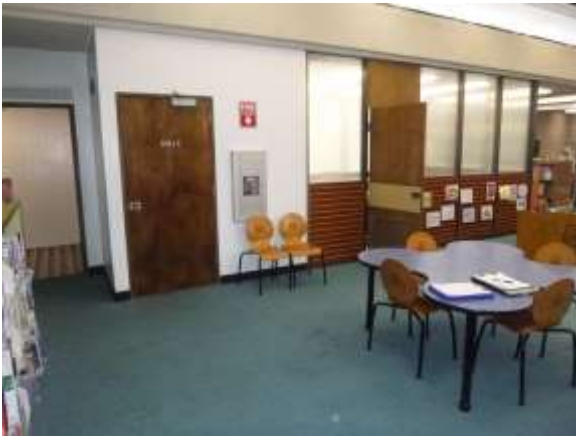
0001047a 4/24/2018 Old wood doors, knobs, missing Braille, and carpet squares Second floor, library, south side
