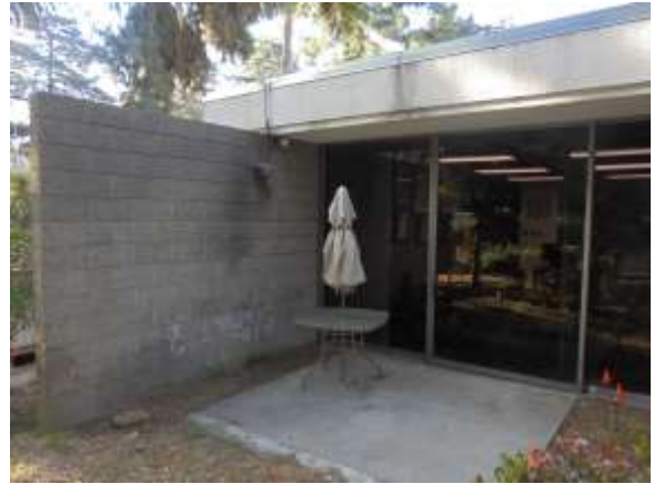
0001004e 4/24/2018 Exterior lighting Building exterior
