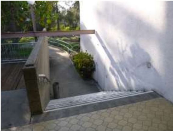
0001016a 4/24/2018 Noncompliant and missing handrails and stucco siding East side steps at main entrance
