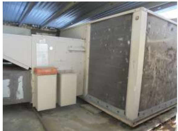
0001036e 4/24/2018 Rooftop package unit #4 Roof
