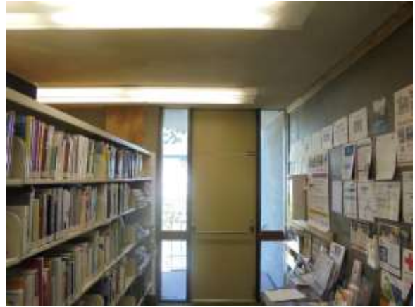
0001058e 4/24/2018 Lack of exit sign and emergency light Second floor, reading room
