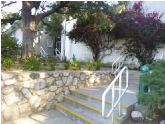
0001024a 4/24/2018 Missing freestanding handrails Southeast sidewalk, south entrance
