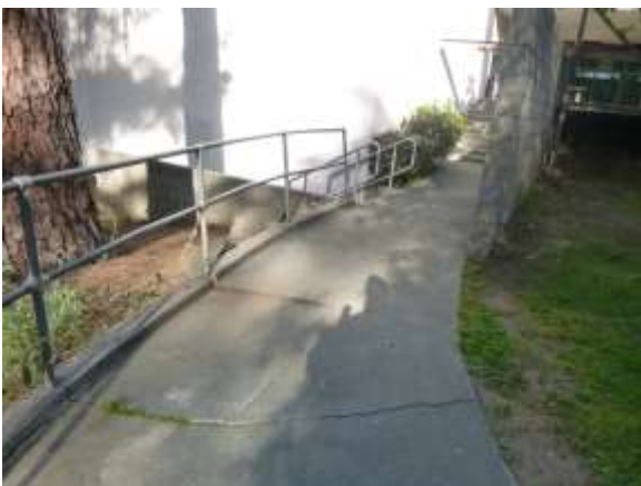
0001021a 4/24/2018 Cracked, sunken sidewalk and leaning and corroded handrails East side of building
