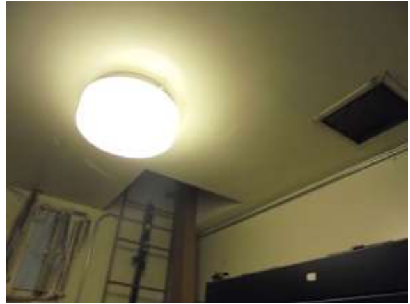
0001040e 4/24/2018 Interior lighting Second floor, IT room
