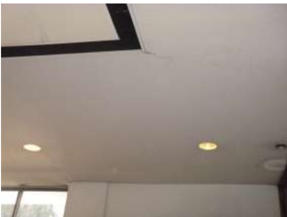
0001051a 4/24/2018 Cracks in painted ceiling and some staining Second floor, library, east side
