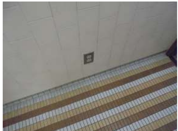
0001082e 4/24/2018 Non-GFCI receptacle Second floor, men's restroom
