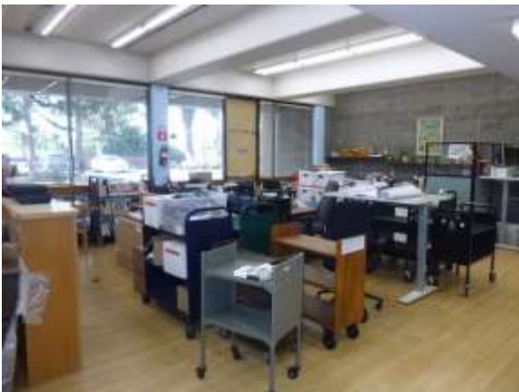
0001069a 4/24/2018 Laminate floor, painted ceiling, and missing LED exit sign First floor, technical services room
