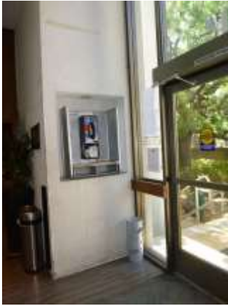
0001074a 4/24/2018 In-wall public telephone, laminate floor, and door operator South entrance to split-level floor
