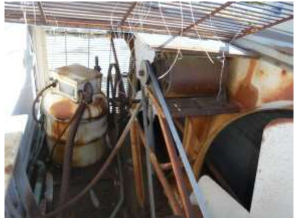
0001029e 4/24/2018 Rusted blower section of rooftop package unit #1 Roof
