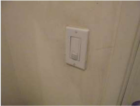
0002020e 4/24/2018 Occupancy sensor Men's restroom
