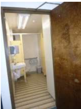
0001048a 4/24/2018 Scarred wood door and ceramic tile floor and walls Second floor, women's restroom
