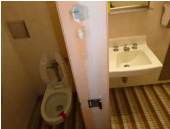
0001072a 4/24/2018 Old restroom fixtures and ceramic tile floor and walls First floor, men's restroom
