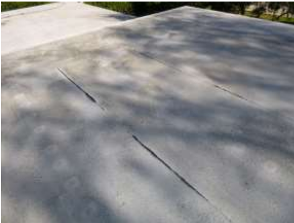
0001035a 4/24/2018 Exposed seams in roll asphalt roof Roof, west side
